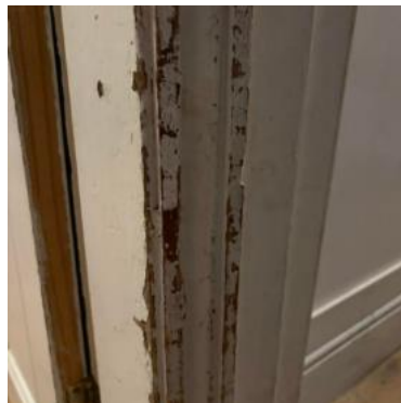
Damaged doorframe from pushchairs
