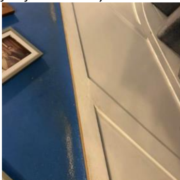
Worn paint on staircase wall
