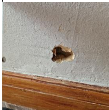
Damage to wall by child
