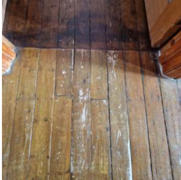
Worn floorboards from high footfall in hallway
