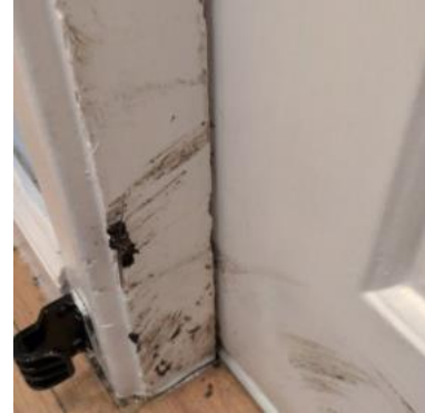
Damaged doorframe from pushchairs
