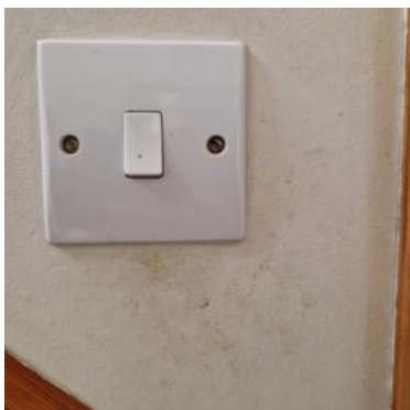
Paint damage around light switch
